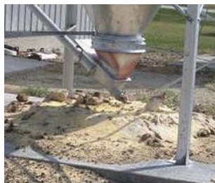
Figure 1. Feed spillage under a feed bin.
